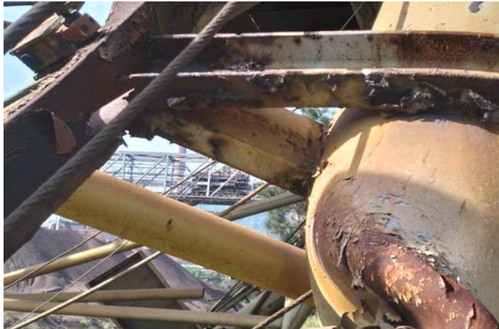
Figure 8. Detailed position of the small ductile breaks of a broken portal crane section
