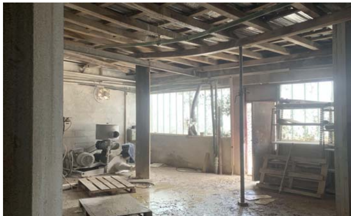
Figure 9. Position of the wooden and steel section supports to plastically deformed sections
