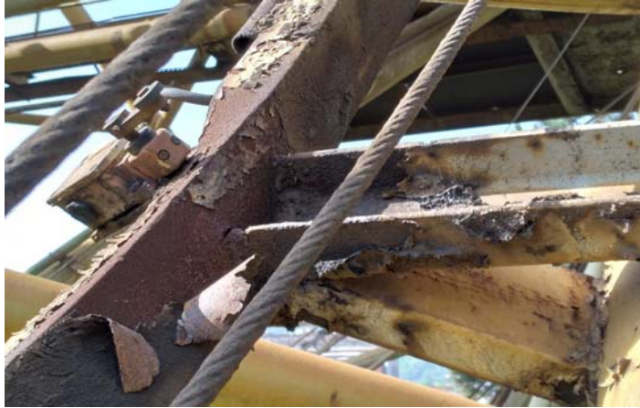
Figure 7. Detailed position of a welded and deeply corroded section of a broken portal crane
