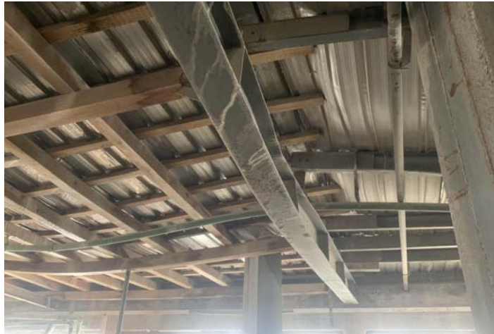
Figure 10. Another position of the wooden and steel section supports to plastically deformed sections
