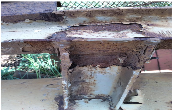
Figure 6. Detailed position of a deeply corroded section of a broken portal crane
