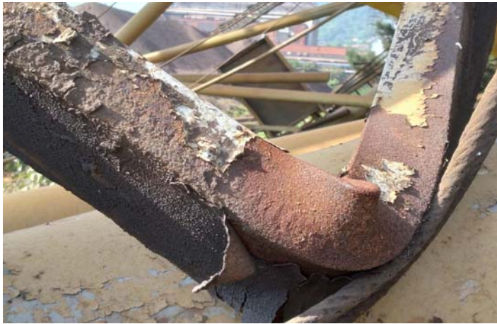
Figure 5. Detailed position of heavy bended section of a broken portal crane
