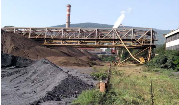
Figure 2. A broken sort of portal crane
